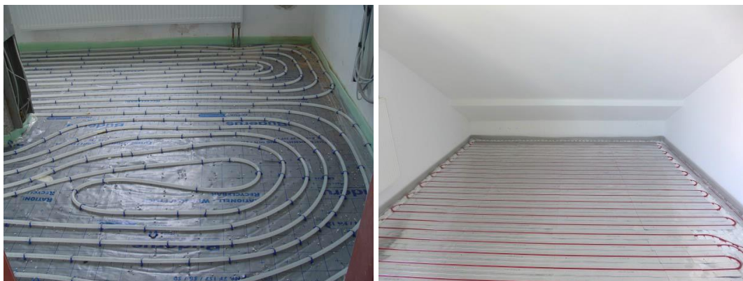
Figure 24: Spiral pipes of the dining room in the ground floors (left) and the child 2 rooms' serpentine pipes in the attics' (right) underfloor heating during installation.
