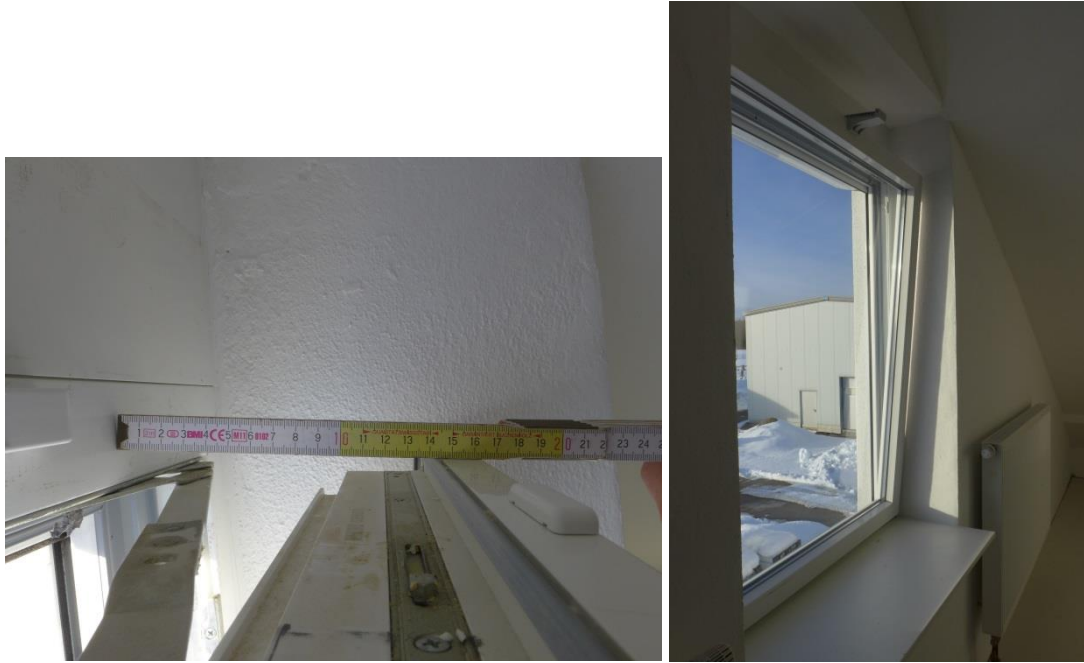
Figure 12: Operated external window in tilted position.
